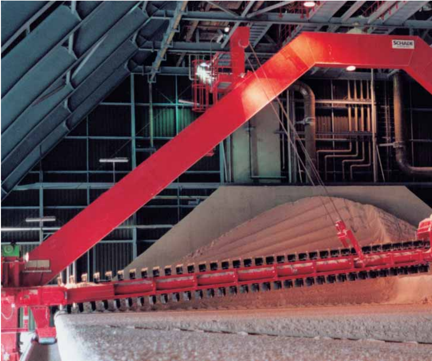
Portal Scraper Reclaimer, 32 m span, 400 t/h, FGD-gypsum
