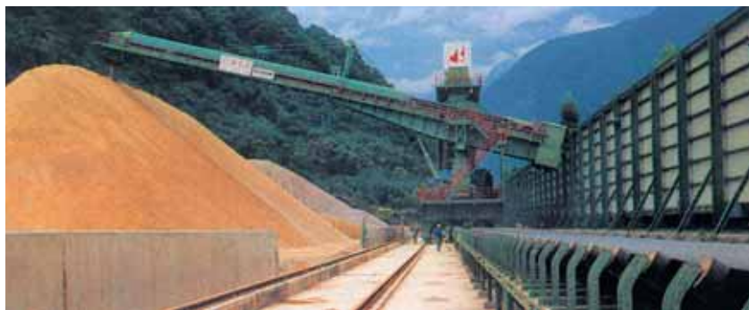
Fig. 3 Luffing Stacker for 2,000 t/h limestone
