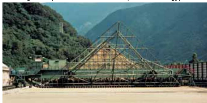
Bridge Scraper Reclaimer, 56 m span, 1.200 t/h, limestone
