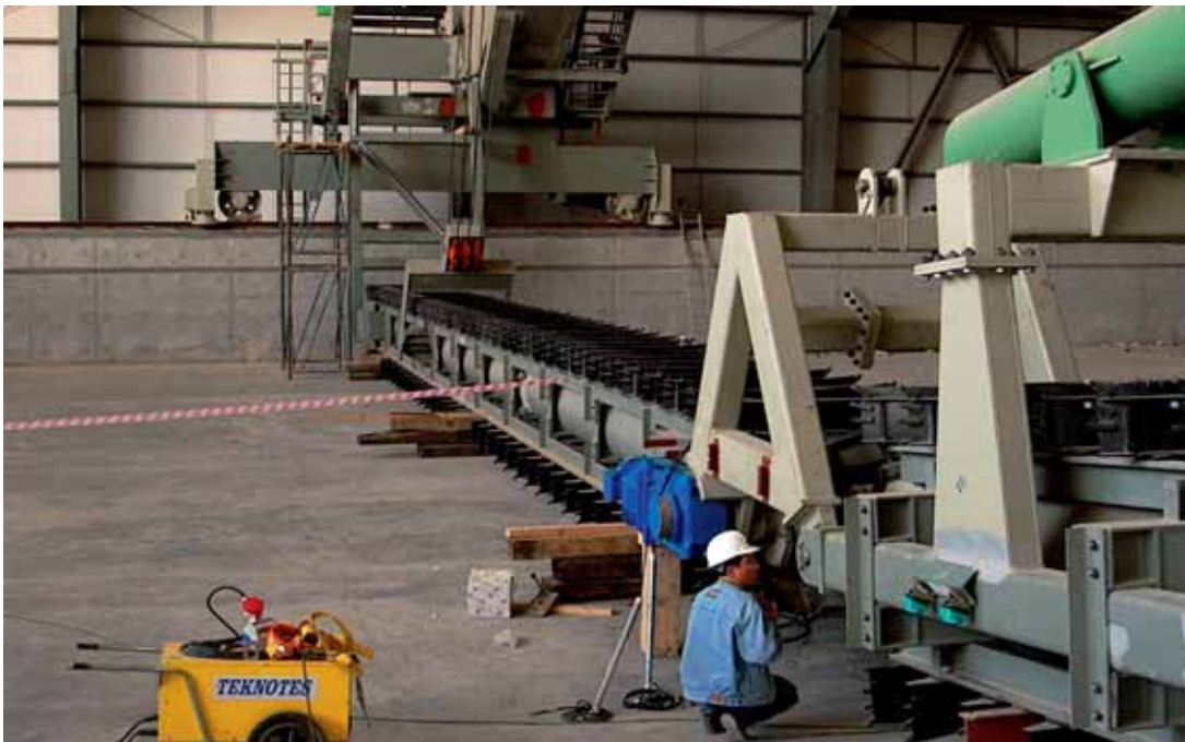
Retrofit situation during capacity increase
