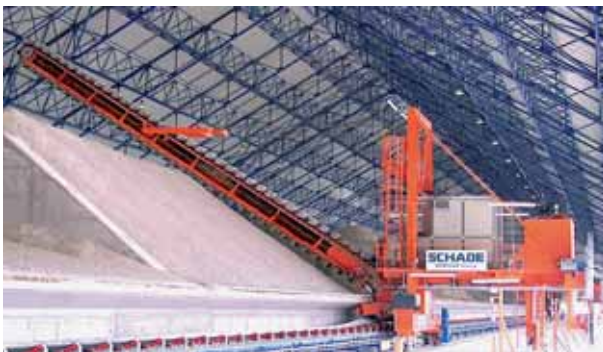
Cantilever Scraper Reclaimer, boom length 18 m, 200t/h, additives
